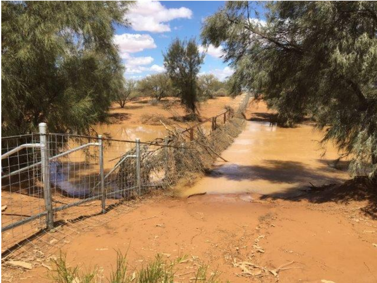
Newly constructed vermin fencing – Sanford River crossing on the western boundary of Meka Station after rains in March 2021
